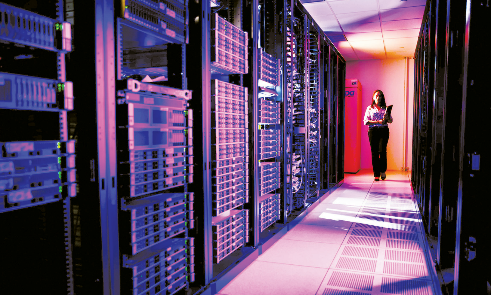
Hotwire Communications server room in Fort Lauderdale
